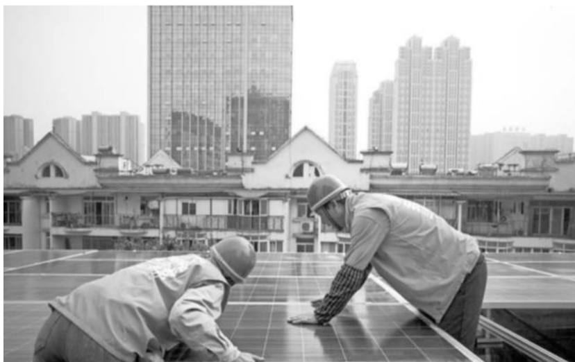
Workers installing solar panels on a roof in Wuhan, China. Greenpeace estimates that in 2015, China covered the equivalent of one soccer field every hour with solar panels.
